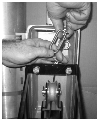
Cable from the LT-4 is attached to the camera lowering cable. Then the camera cable is disconnected from the eyebolt (cable parking stand).
